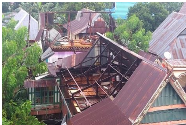
Fig 2. Sample of roof damage
