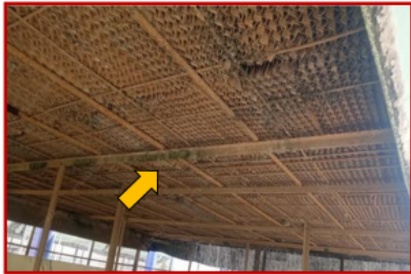
Majority of the area cooling tower fins and nozzle pipelines are choked
