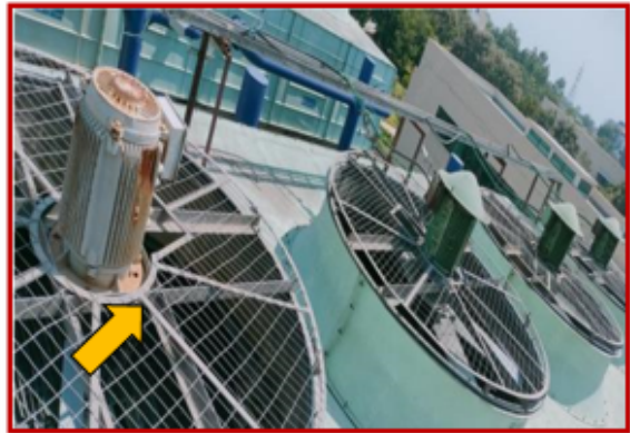
Cooling Tower Fan motors winding failed and fan blades damaged/bearings are failed
