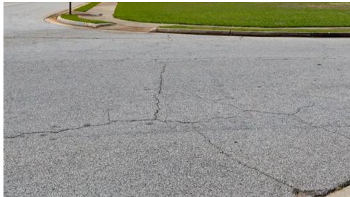
Fig 1: Reflection Cracking of Asphaltic Overlay
